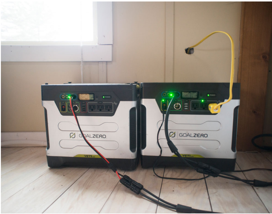
The Busbys utilize two Goal Zero Yeti 1250 Solar Generators as power and energy storage for their yurt.
